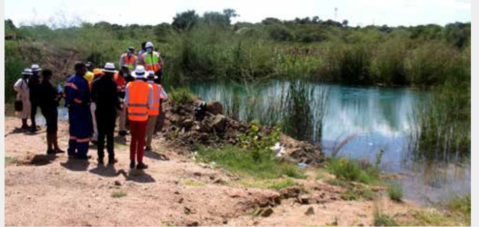
Water Utilities Corporation (WUC) briefed the media on the planned shut down Oodi-Mmamashia North South Carrier pipeline to fix a major leak on the pipeline. The shutdown will start from 24 March until 26 March 2022, resulting in water supply interruption in Mochudi, Lobatse, Gaborone and surrounding areas. WUC chief executive officer Gaselemogwe Senai briefed the Media at site where the fixing will take place. (Pic:PRESS PHOTO)
